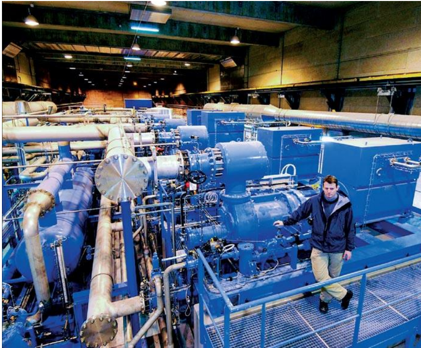
Compressor unit of the 4.5 K refrigerator
